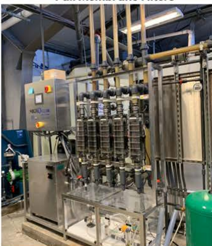
Chlorine Generation System
